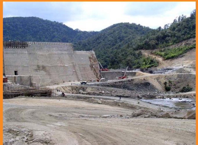
Chalillo Hydroelectric Project under construction. The project is scheduled for completion in June 2005, with commissioning of the Powerhouse in September 2005.
